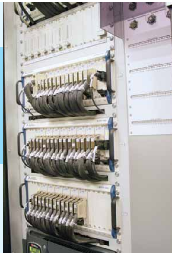
Figure 6 - PXI-based Fault Insertion System (photo by courtesy of Clemessy)
